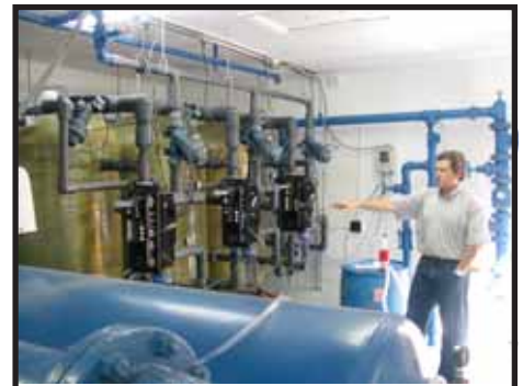
System Owner Eric Thomas explaining the function of computer controller automating system operation.
