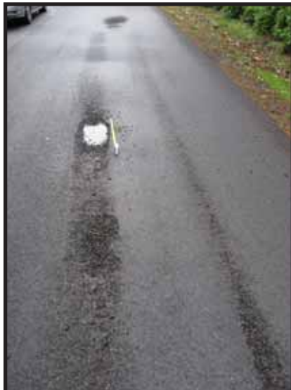
Area on Kala Point Drive where overlay is failing.
