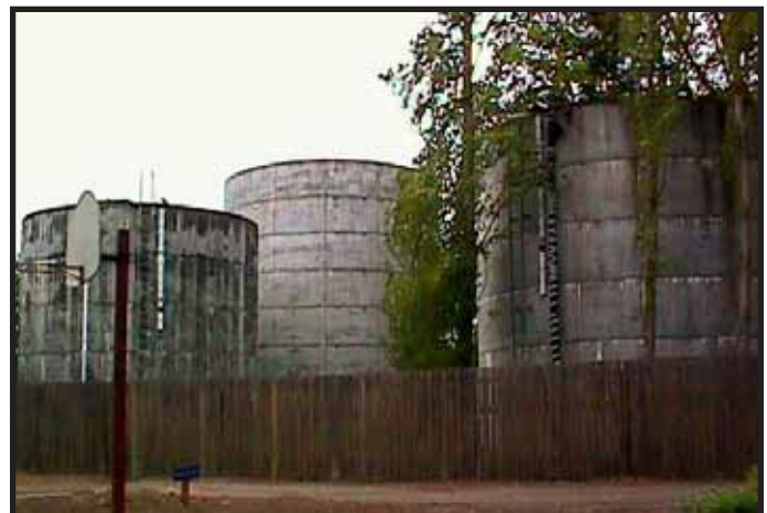
Kala Point Water Tanks off Pinecrest
